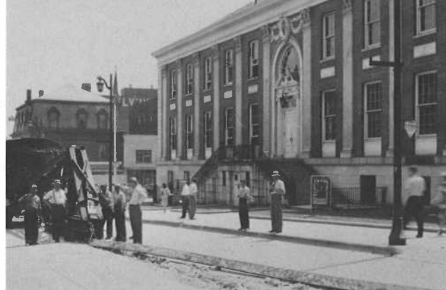
Trolley tracks are removed for scrap in Burlington in 1943. Photo by L. L. McAllister. Courtesy of Special Collections, University of Vermont Library.
